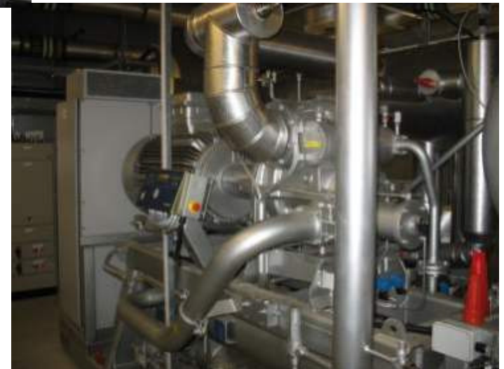
PRD High Wycombe, UK Ammonia Chillers
