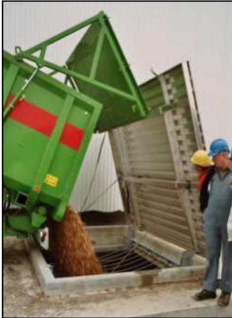
Cilag, Schaffhausen, Switzerland Wood Chip Boiler 350 kW boiler
