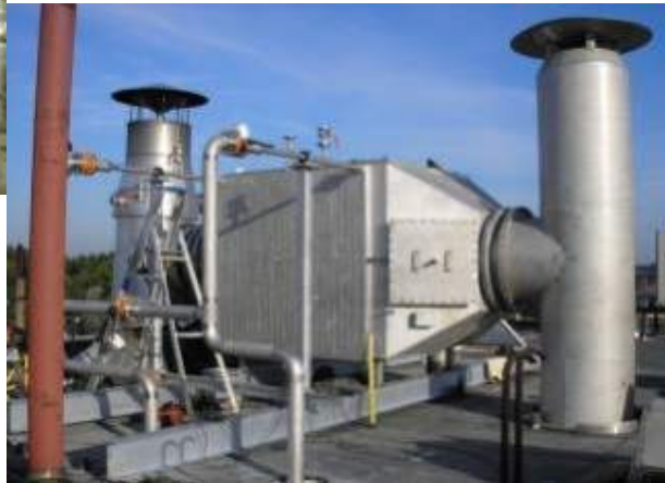
Janssen Beerse, Belgium Stack Gas Economizer
