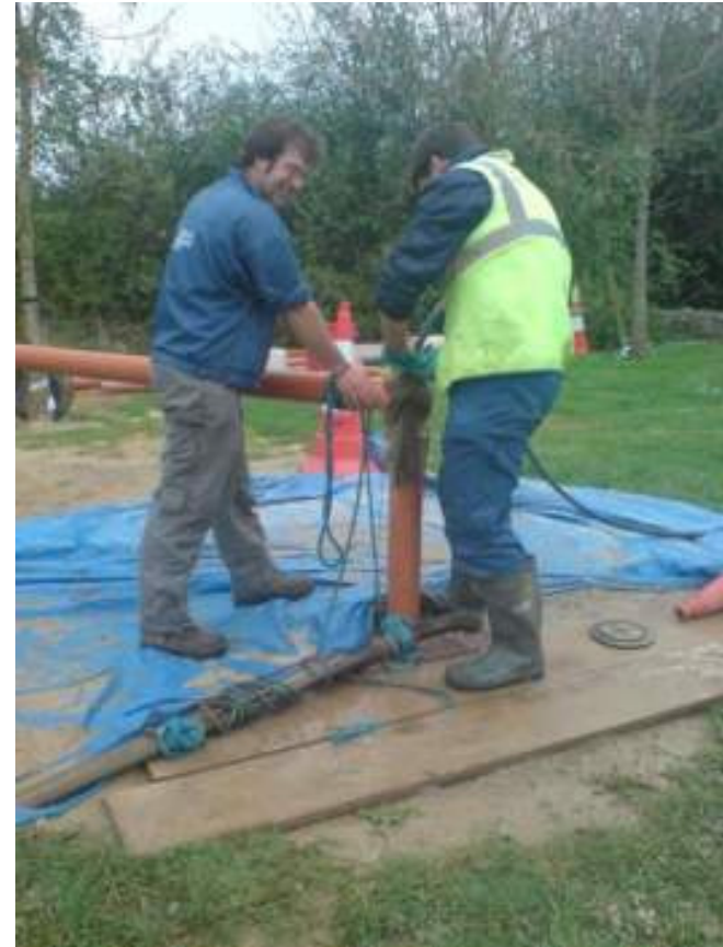
Vistakon – Limerick, Ireland Geothermal Cooling System
